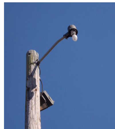
Existing light pole
