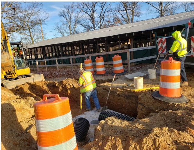
Stormwater Management Improvements
