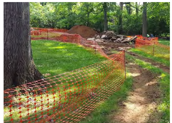
Figure 53: Tree protection fencing during trail construction
